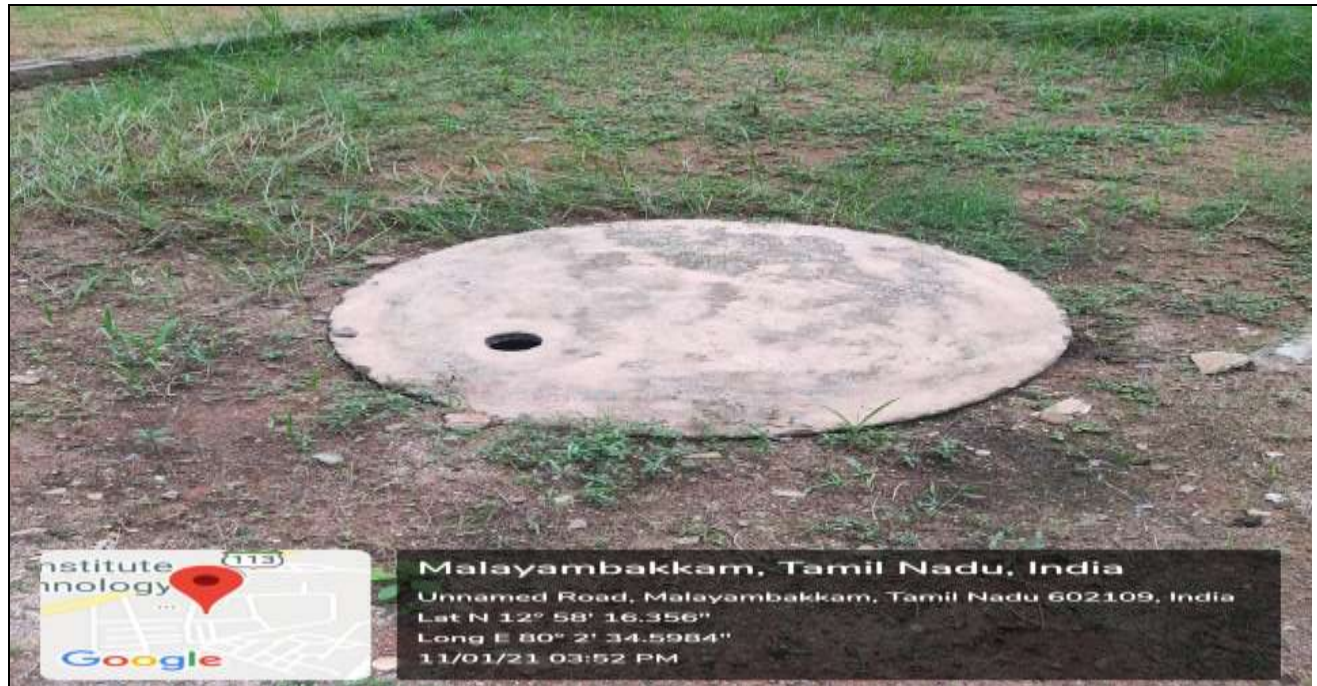
Rain water harvesting collection points
