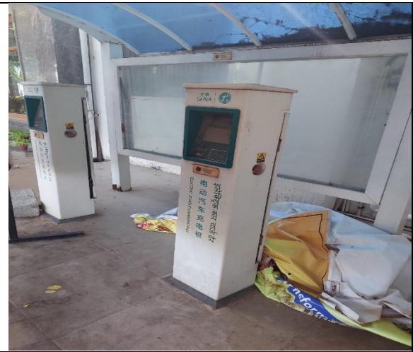
Charging points for EV
