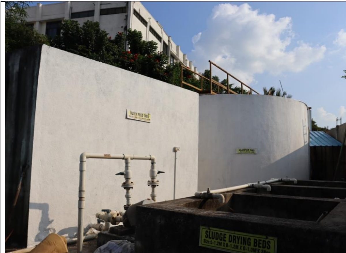
Filter Feed, Clarifier and Sludge drying Beds
