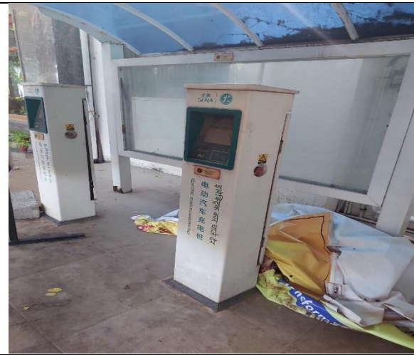
Charging points for EV
