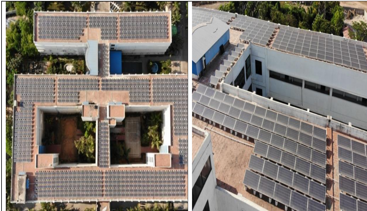
Roof Mounted Solar Panels (Chennai Institute of Technology)
