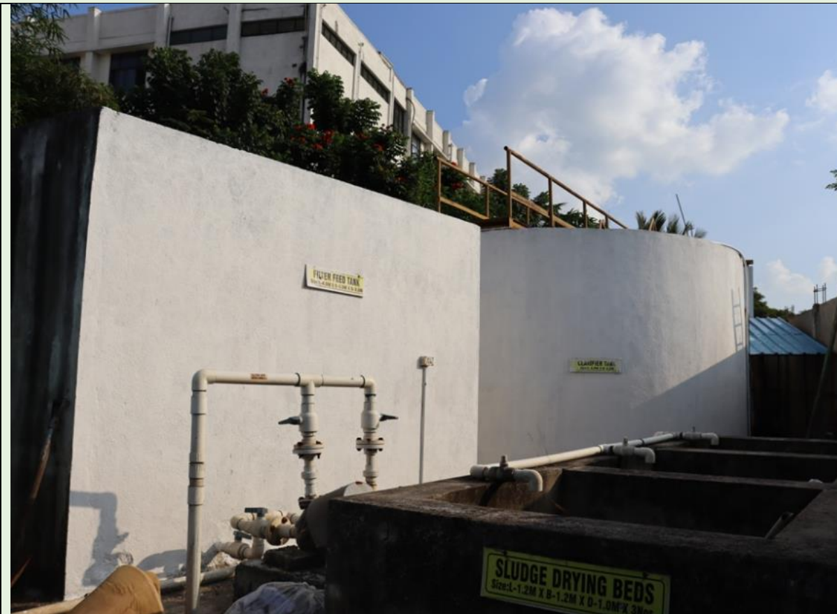
Filter Feed , Clarifier and Sludge drying Beds
