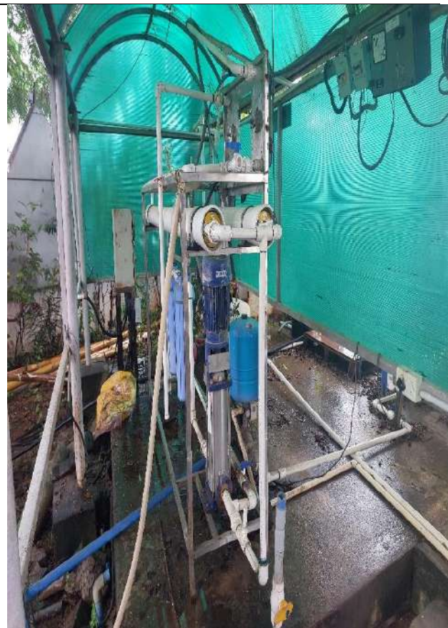
RO System Unit Covered By
