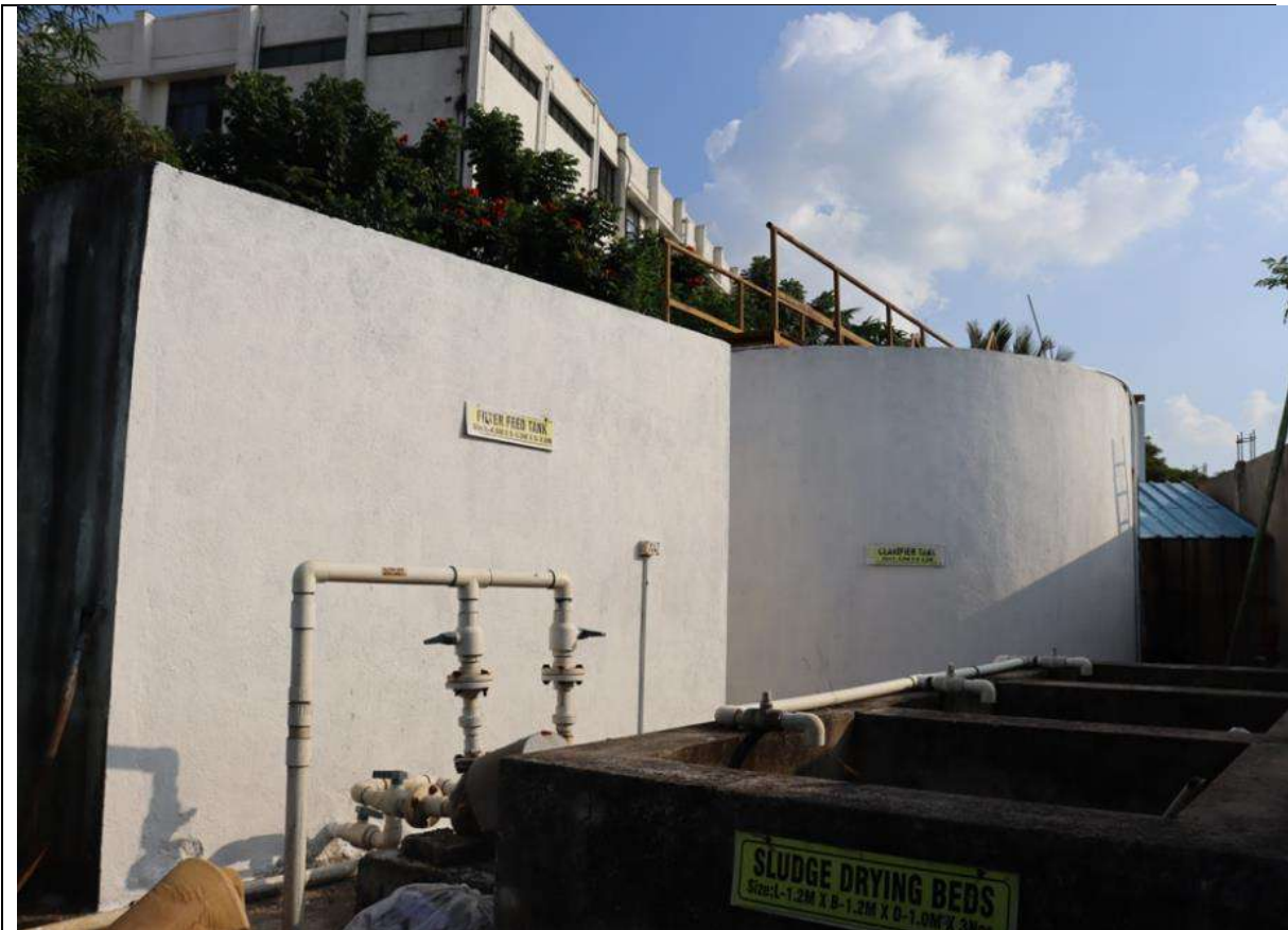
Filter Feed , Clarifier and Sludge drying Beds
