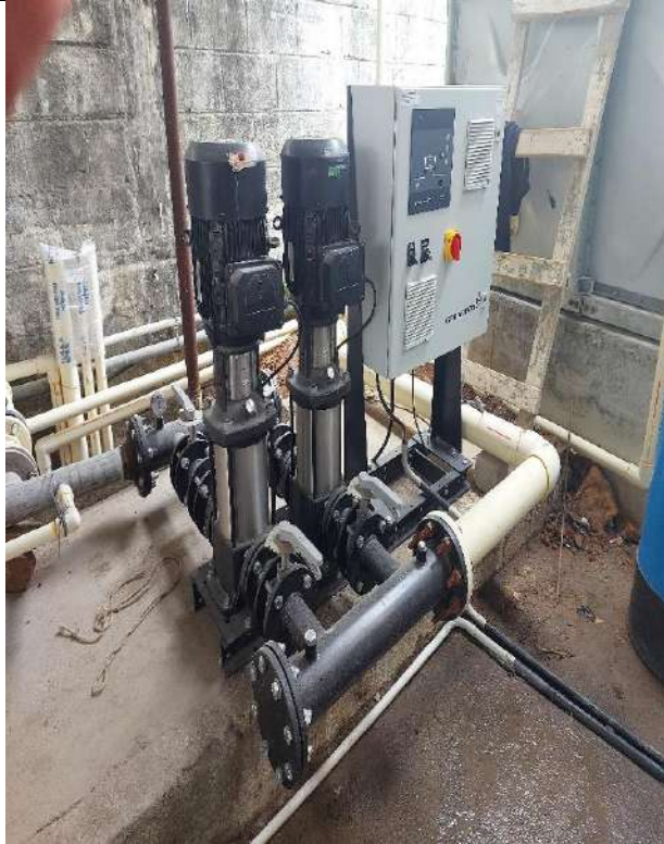
System provided with Adequate clearance
